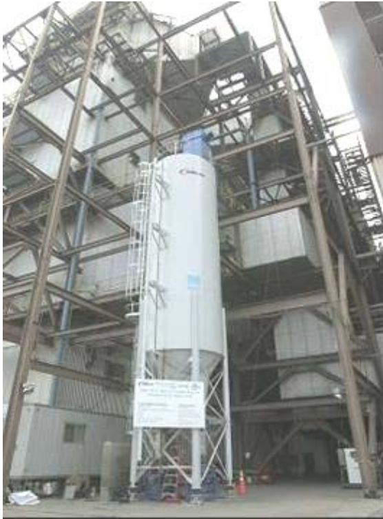
Activated carbon silo
