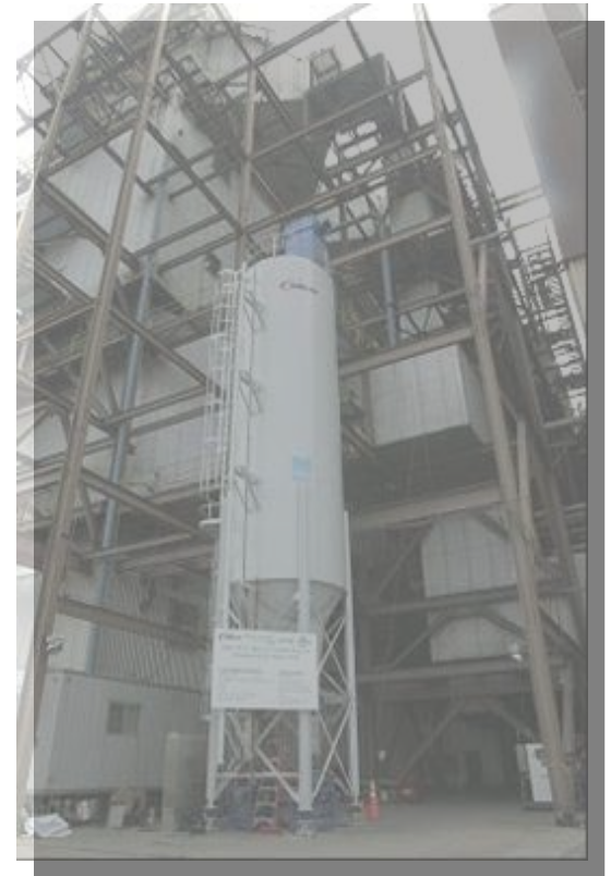
AC Storage Vessel
