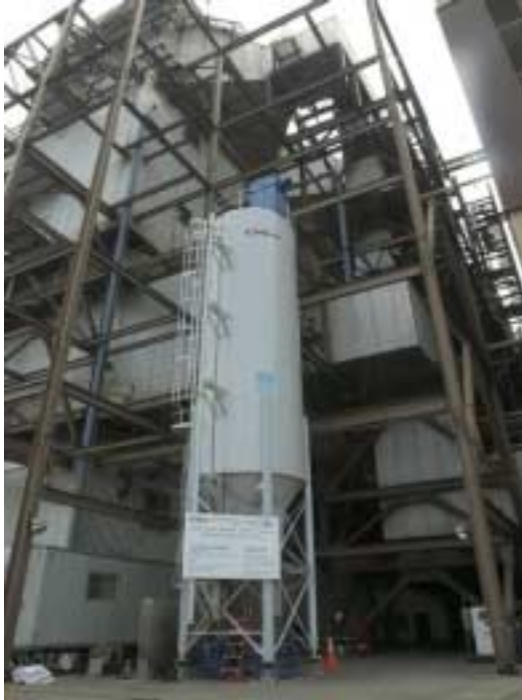
Sorbent Injection System at WEPCo Pleasant Prairie Station
