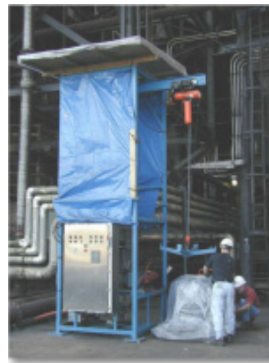
ADA sorbent feed system at the Gaston power plant
