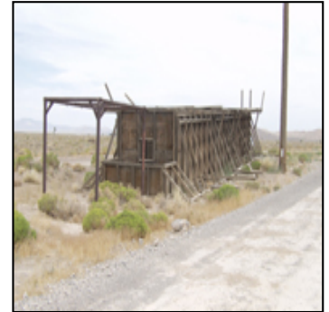
This angle of the structure depicts the south and west elevations, with an additional pole façade on the right side.
