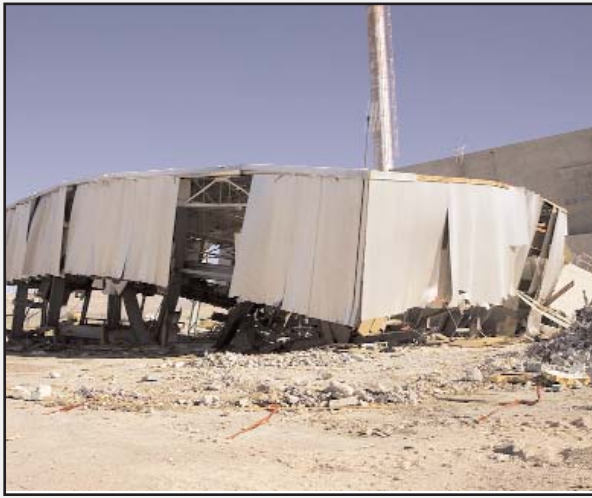
Now on the ground, the steel and concrete from the controlled demolition can be handled safely for disposal at the landfill.
