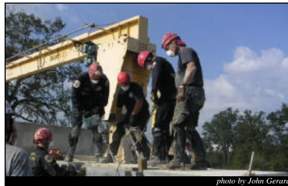
NTS Technical Rescue team members Chris Swiger (middle jackhammer) and Kerry Mackey (far right), along with other course attendees, make a downward penetration into a vault simulating a pancaked structure during the training course.
