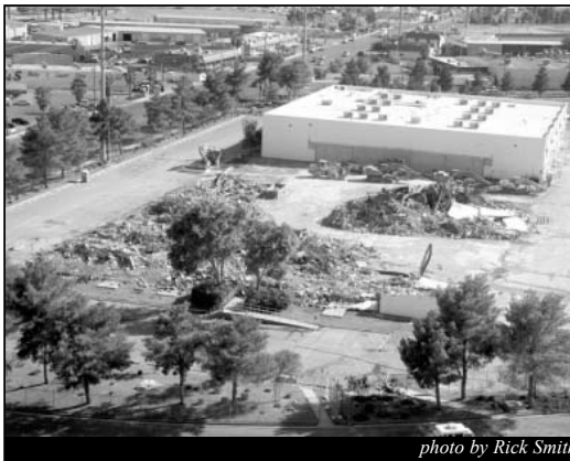
Piles of rubble replace what were once buildings B-1 and B-2.
