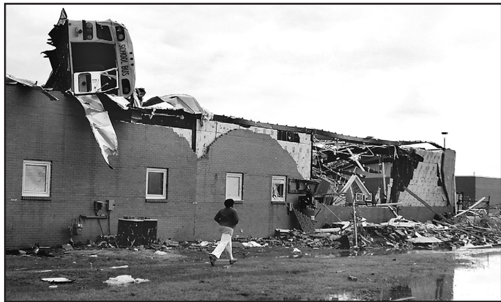
Figure 7-2. A school bus was lifted atop a section of Caledonia High School, Caledonia, Mississippi (January 2008)
