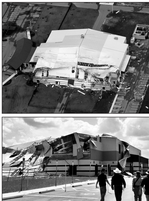
Figure 1-3. Severely damaged hurricane shelter at Turner Agri-Civic Center, Arcadia, Florida (2004)
