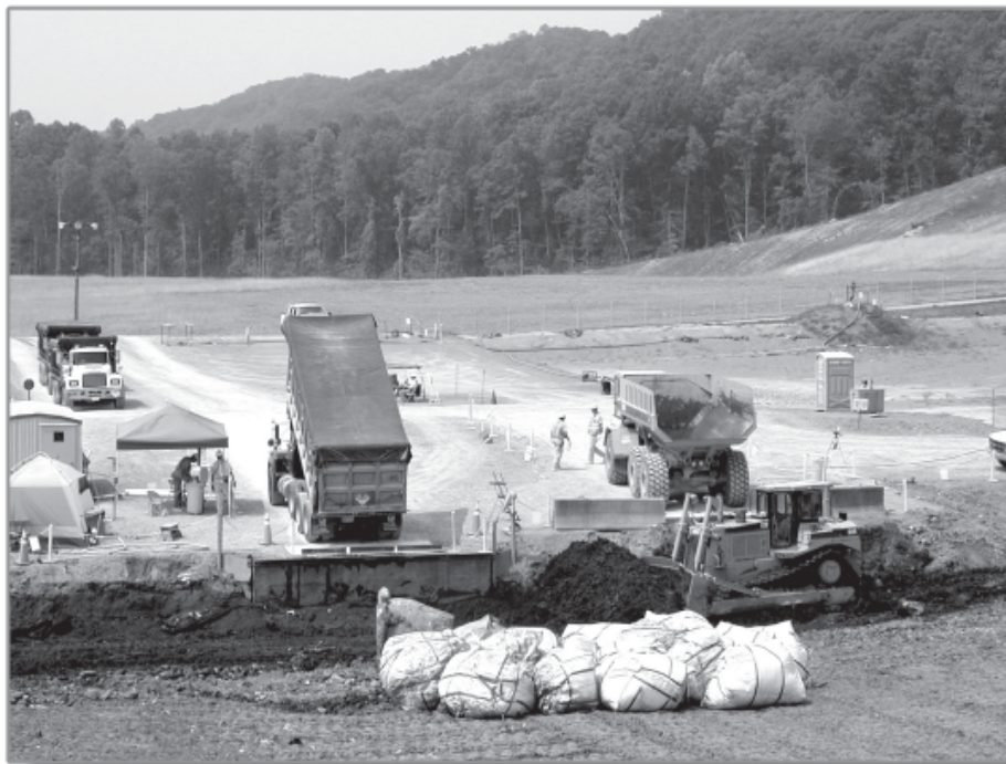
Part of the Oak Ridge Reservation cleanup plan is to unearth problem wastes and relocate them to new, well-designed disposal facilities on the reservation. This photo shows wastes from a cleanup project being disposed in the new Environmental Management Waste Management Facility at Y-12. The facility was designed to minimize the possibility of wastes leaching into the environment by enveloping them above and below in many layers of synthetic and natural liner materials.
