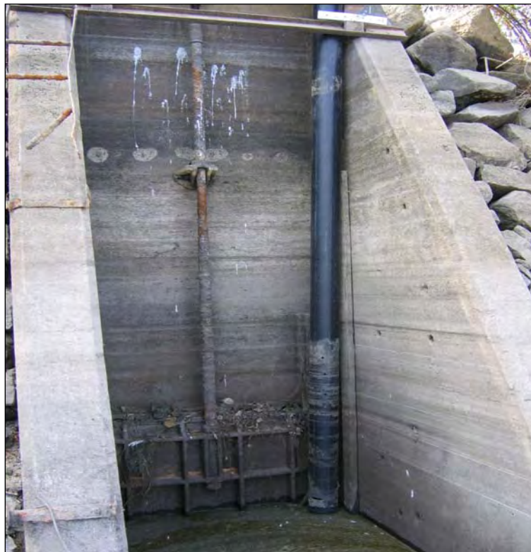
Figure 4. EDS 6600 Installation at the Lake O'Neill Outlet, October 5, 2006.
