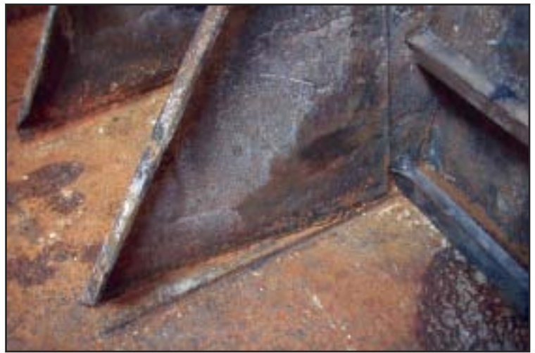
Figure 6a. Close-up of tripped toe bracket. USCG photo.
