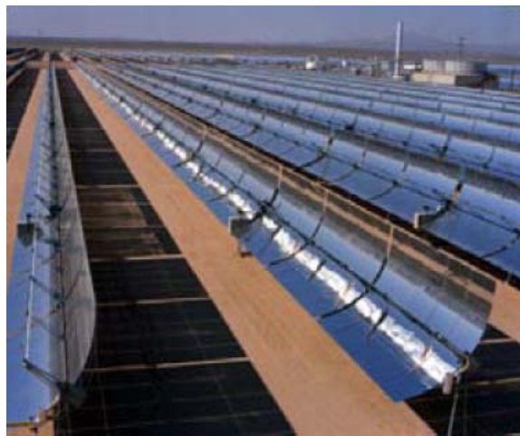
Figure 1.8. Parabolic Trough System
