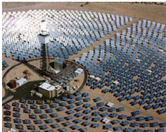
Figure 1.10. Power Tower System
