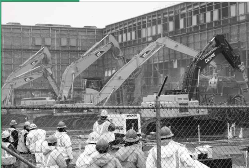
Track-driven excavators began taking apart the historic K-25 Building at East Tennessee Technology Park on December 16, 2008.
