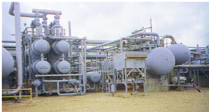
CO 2 separation facilities at Little Creek field.
