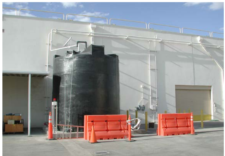
Figure A-4. Storage tank used to hold discharge water from the active dewatering wells on the north side of Building A-1. (Photo by S. L. Drellack, August 9, 2006)
