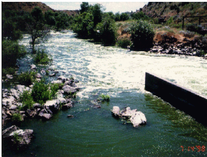
Figure 20 - View looking downstream along the east wall of the outlet works stilling basin.
