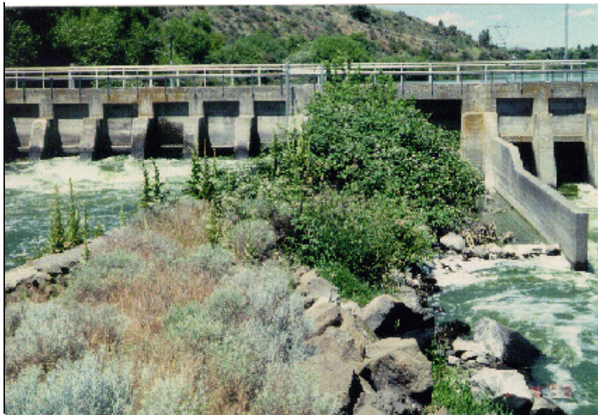
Figure 18 - View looking upstream at Keno Canal and the west outlet works stilling basin wall.
