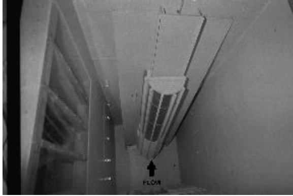
Figure 8. —Photograph of existing intake configuration (modification one).
