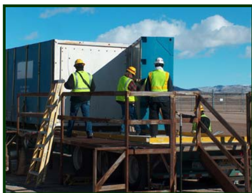
Workers offload ULWBR material from Idaho National Laboratory at the NTS Radioactive Waste Management Site.
