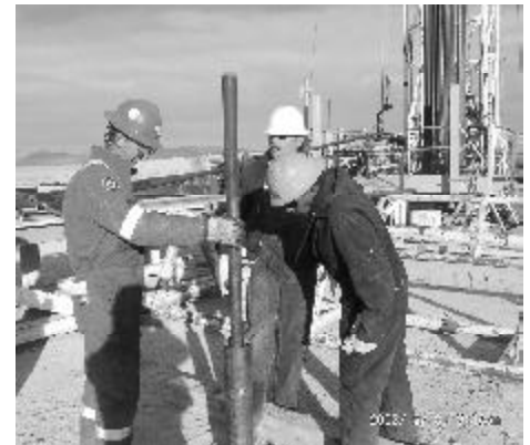
UGTA gets to work in the field: crew runs submersible pump in a well.
