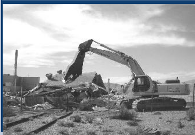
Heavy equipment known as Hydraulic Shears were used at the R-MAD decontamination facility to safely dismantle the structure.
