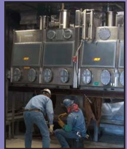
Workers prepare the glovebox for removal from the Visual Examination and Repackaging Building.
