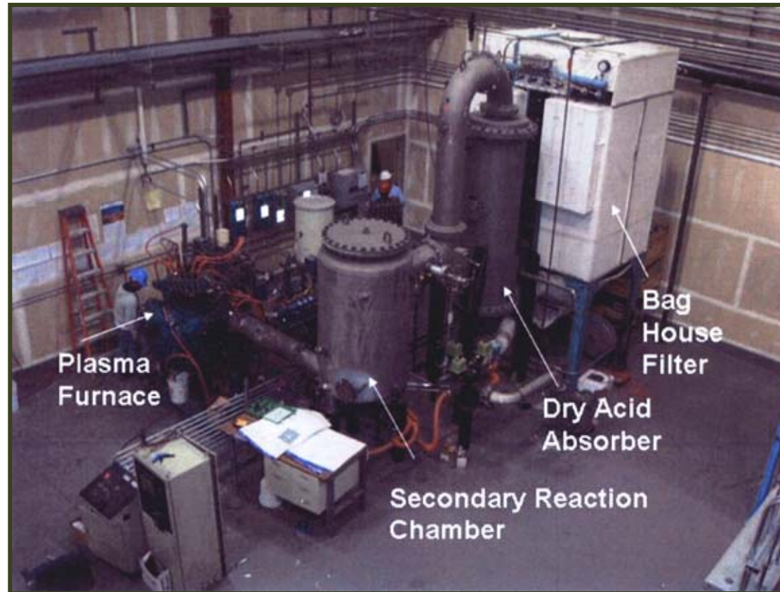
Unit at PermaFix Northwest
