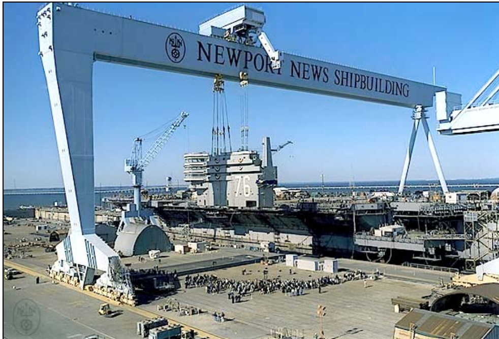
Figure M-1. Lifting the Island for the USS Ronald Reagan, CVN 76 (excerpted from www.nn.northropgrumman.com/photogallery )
