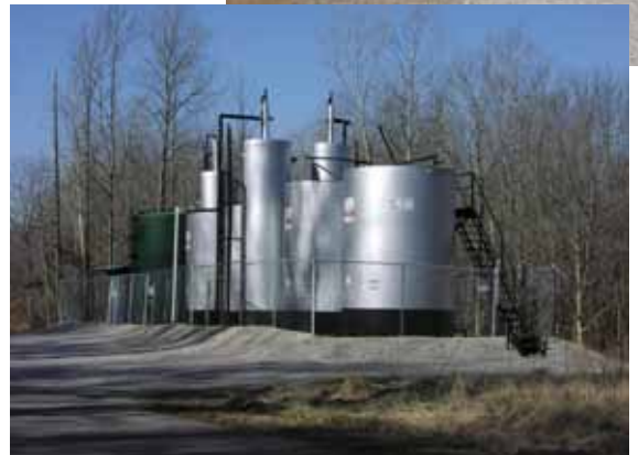
After drilling, the site is reclaimed, and the well head and fluid separation and/or compression equipment may be all that remain in the rural landscape.
