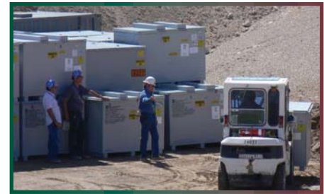
Workers place a metal box containing mixed low-level radioactive waste in a disposal cell at the Area 5 Radioactive Waste Management Complex located in the southeast portion of the Nevada Test Site.
