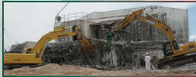
Heavy equipment is used to dismantle Test Cell A - a contaminated facility located in the southwest portion of the Nevada Test Site used for nuclear rocket development during the 1960s.
