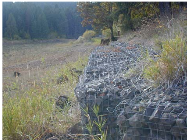
Photo 2-3. Shoreline erosion control structure at Sain Creek Picnic Area (at low pool).
