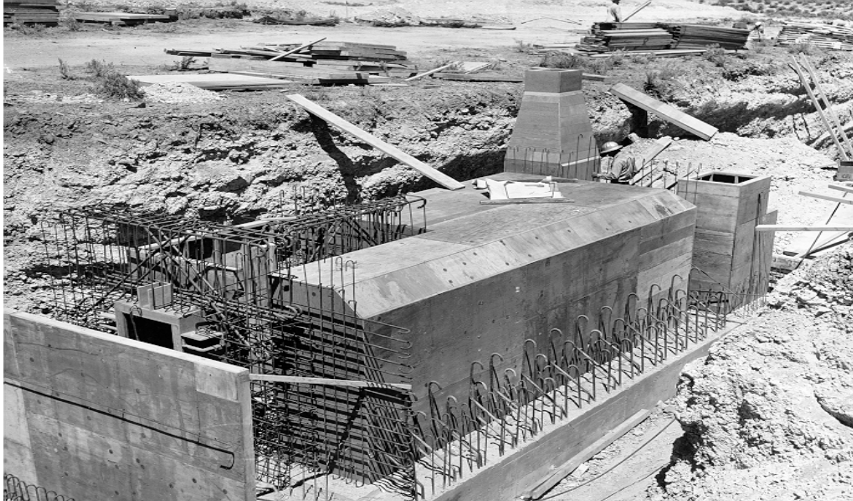
One of nine shelters sponsored by the former West German government. The main room had a capacity of 25 people. At the left foreground is the location for the stairwell and main blast door. The shelter measured 9 feet by 21 feet by 72 feet. The walls and roof were two feet thick.
