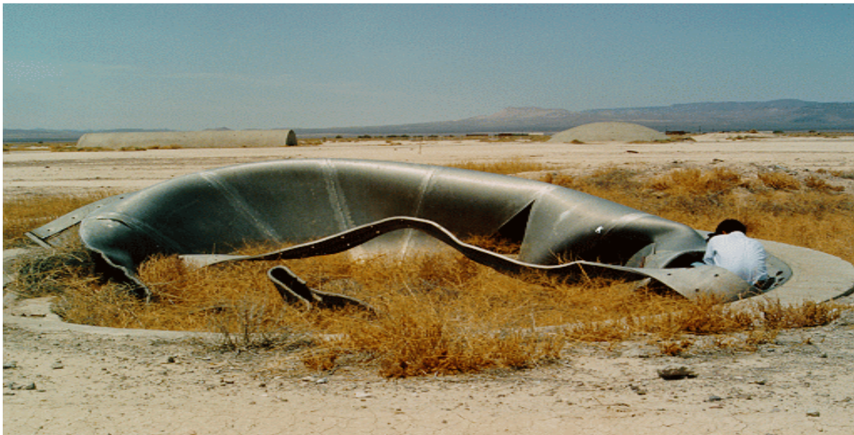
One of two collapsed aluminum shelters.
