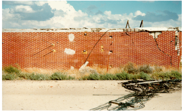
Windowless modular structure after the test. Notice the displacement of the wall.
