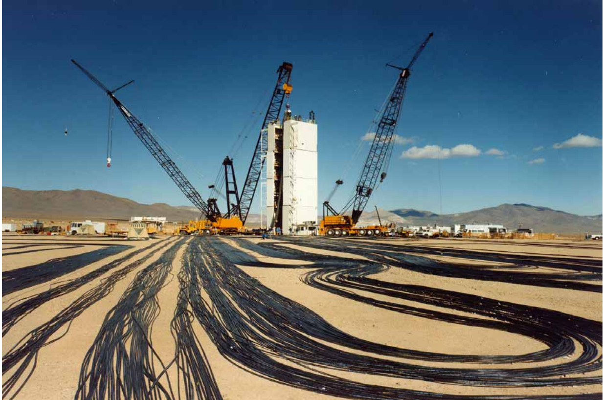
Signal cables are laid out at a former test location on Yucca Flat.
