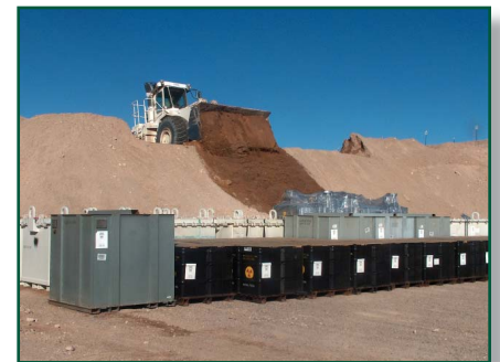
Low-level waste boxes are covered with native soil following disposal at the Nevada Test Site.
