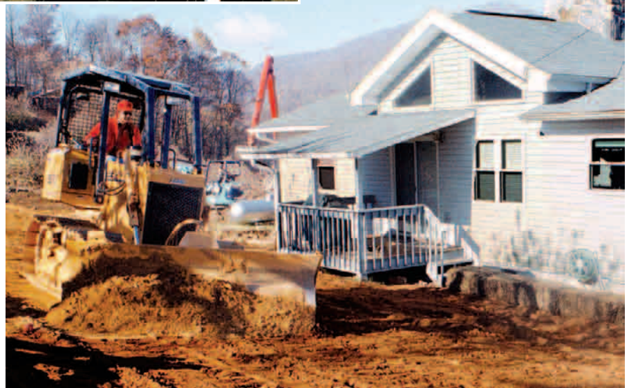
Landscaping. A bulldozer scrapes a layer of contaminated soil from a yard in the Barber Orchard subdivision in North Carolina, once the site of a large apple orchard. Due to contamination with former agricultural chemicals, the subdivision was designated a Superfund site in 2001. EPA-supervised cleanup, mainly by removing soil, is on hold pending further funding.
