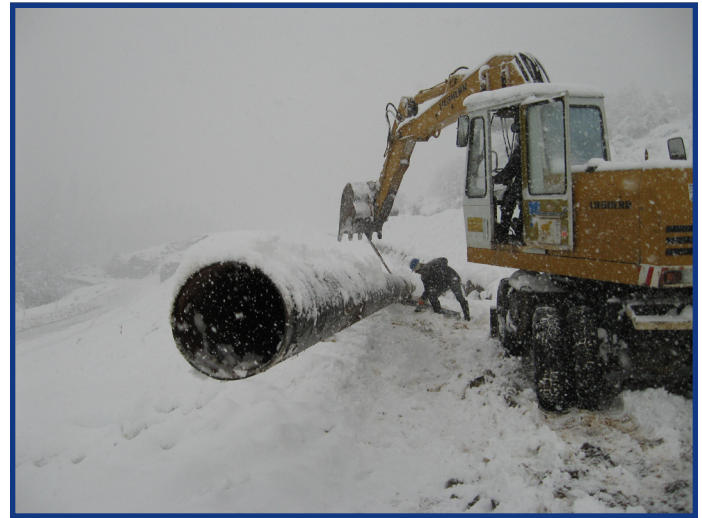
Poti's distribution system is badly rusted and damaged. MCC will fund, among other projects, emergency repairs to the existing water transmission pipeline and rehabilitation of Poti's water distribution network, which is 90% completed.
