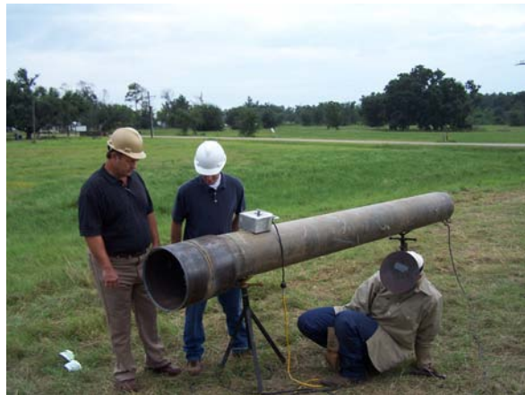
SPR personnel monitoring a Welder Qualification Test for the Raw Water Pipeline replacement job.
