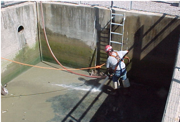
At SPR a Maintenance Technician cleans the site's retention pond 2, as part of DynMcDermott's Preventive Maintenance Program.
