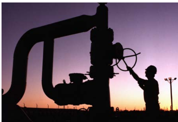
A wellhead at the SPR Bayou Choctaw Site.
