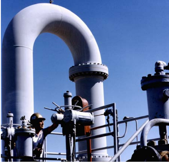
Prover loop on meter skid at the SPR Bryan Mound Site.
