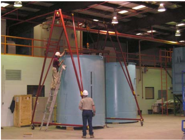
An SSC technician disconnects spreader bar from wastewater tank to make way for new R&D project at NETL-Morgantown.
