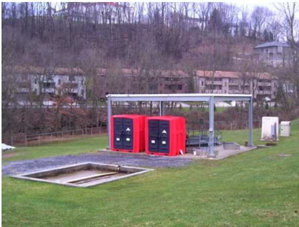
New acid/base enclosures installed at NETL-Morgantown clarifier improve worker safety and reduce the likelihood of spills.
