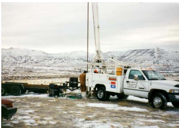
NETL employees install monitor well for ground water at Rock Springs field site.
