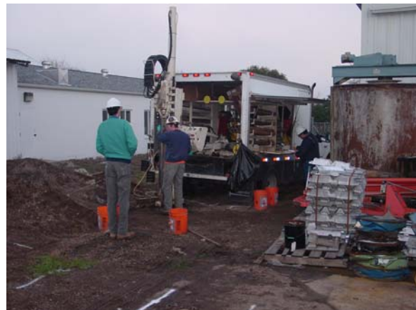
ARC ground water Program Manager, Steve Curfman, oversees the drilling rig during a ground water investigation.
