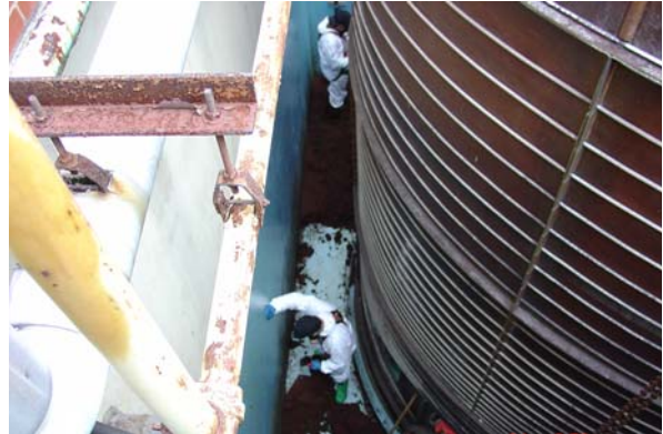
NETL Staff remove flocculent from around the outside of the Equalization Tank at NETL-Pittsburgh for disposal.
