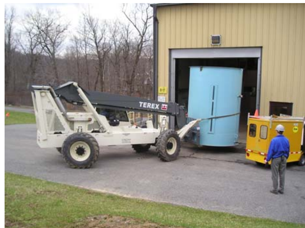
An NETL Safety Engineer looks on as one of four wastewater tanks is removed from Building 17 for safe transport to lay-down area.
