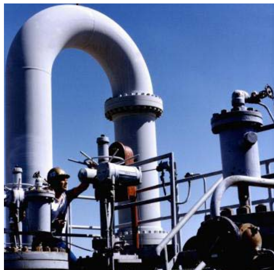
Prover Loop on Meter Skid at SPR's Bryan Mound.
