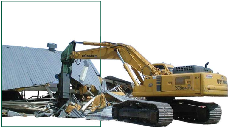
Demolition of the Reactor Maintenance, Assembly, and Disassembly decontamination building at the Nevada Test Site.
