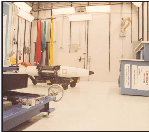
The DAF includes assembly bays for activities involving uncased conventional high explosives and special nuclear material.
