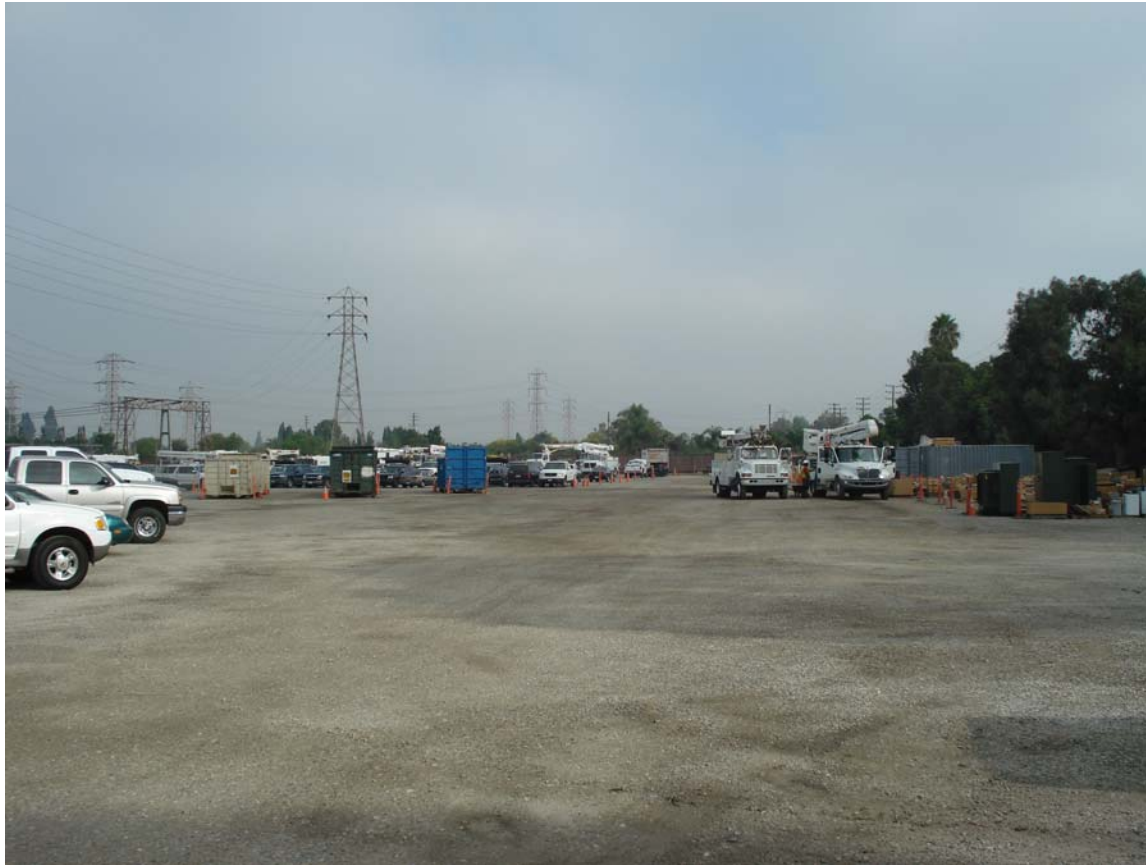
Figure 10: Looking north from southern boundary of the substation.
