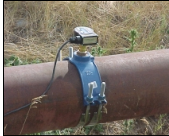
Figure 8.—Vortex shedding meter and flow display which is also on a 10-inch pipeline.
