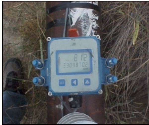
Figure 4.—The paddle wheel flow meter display for the installation in figure 3. The flow rate is displayed in gallons per minute and total gallons.
