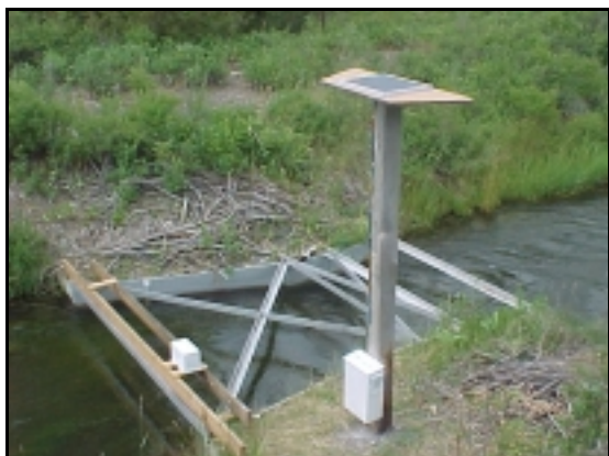
Figure 1.—The open channel flow recorder installed upstream from an 8-foot Parshall flume. The solar panel is mounted on top of the post with the battery below.
