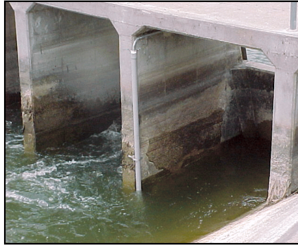
Figure 10.—The transducer is pipe mounted to a concrete structure upstream from a weir wall.
