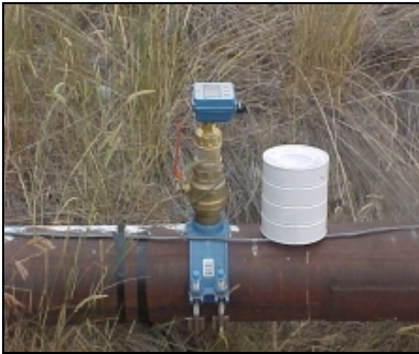
Figure 3.—The paddle wheel flow meter with display installed on an 8-inch pipe in Montana. (The white can is placed over the sensor to shade it from the sun).
