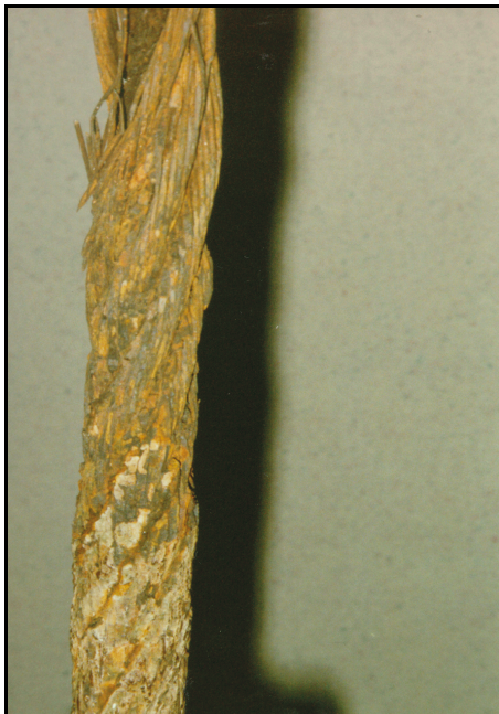
Figure 3.—Stewart Mountain Dam wire rope.
