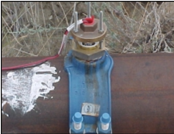
Figure 5.—Another paddle wheel flow rate sensor which is also installed on an 8-inch pipeline.
