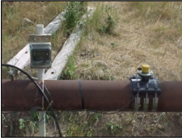
Figure 7.—Propeller flow meter and display installed on a 10-inch pipeline.
