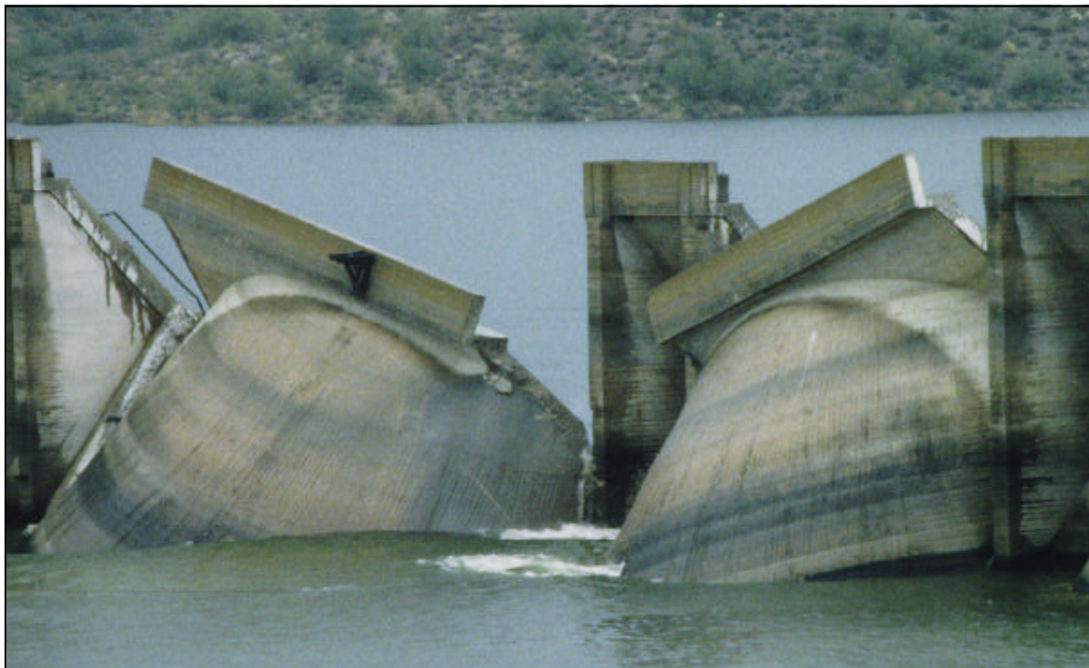
Blocks of concrete at historic Waddell Dam begin to fall away after cuts to create breach.
