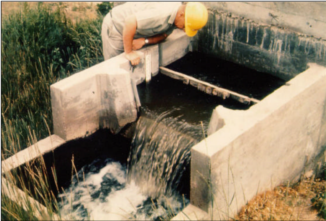
Figure 1.—Weir box turnout with Cipolletti Weir.
