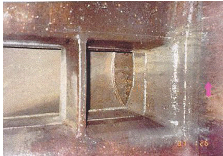
Photograph 5. —Typical view of the air vent inside the river outlets. The arrow indicates the direction of flow. The vents are located on the tube's ceiling immediately downstream of the service gate.
