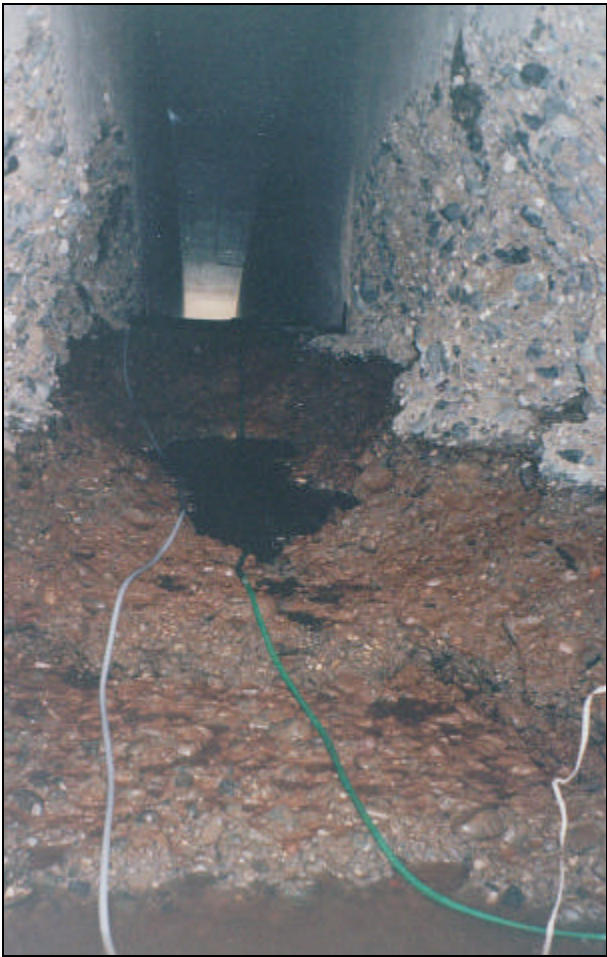
Photograph 3.—Gate 4 cavitation damage downstream of gate liner. Note second bowl-shaped damage downstream of smaller size which clearly indicates cavitation instead of strictly erosion.
