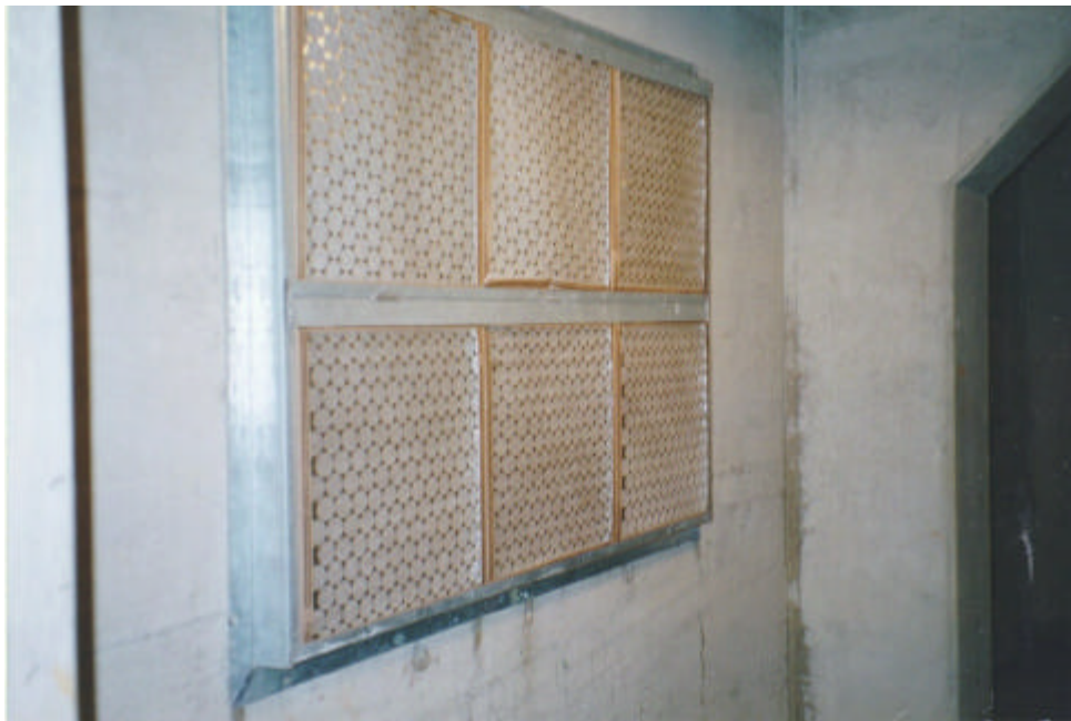
Photograph 2.—Air filters attached to the inside of the louvers.
