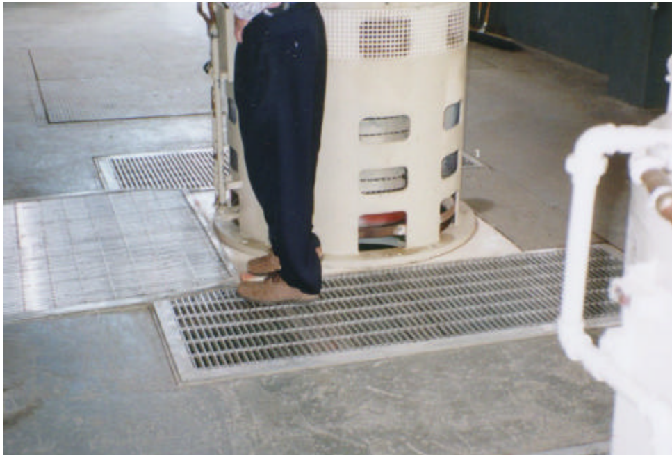
Photograph 3.—Aluminum grating over the floor openings adjacent to the motors.
