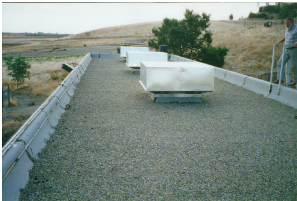
Photograph 4—New roof vent motors atop the pumping plants.
