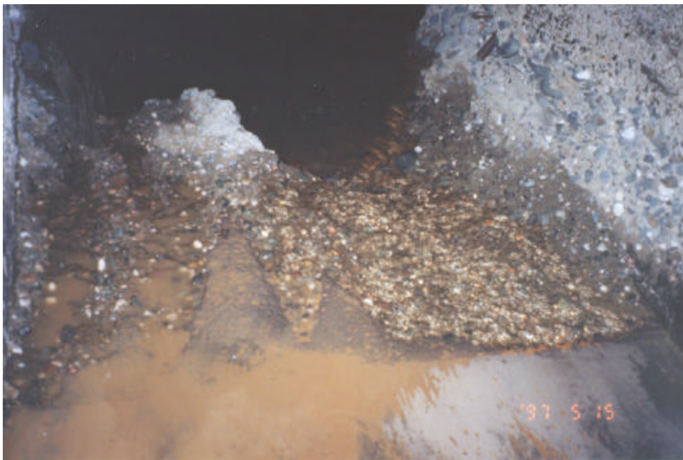
Photograph 2.—Inside river outlet No. 3 looking downstream from the metal liner. Cavitation damage begins at the end of the liner.
