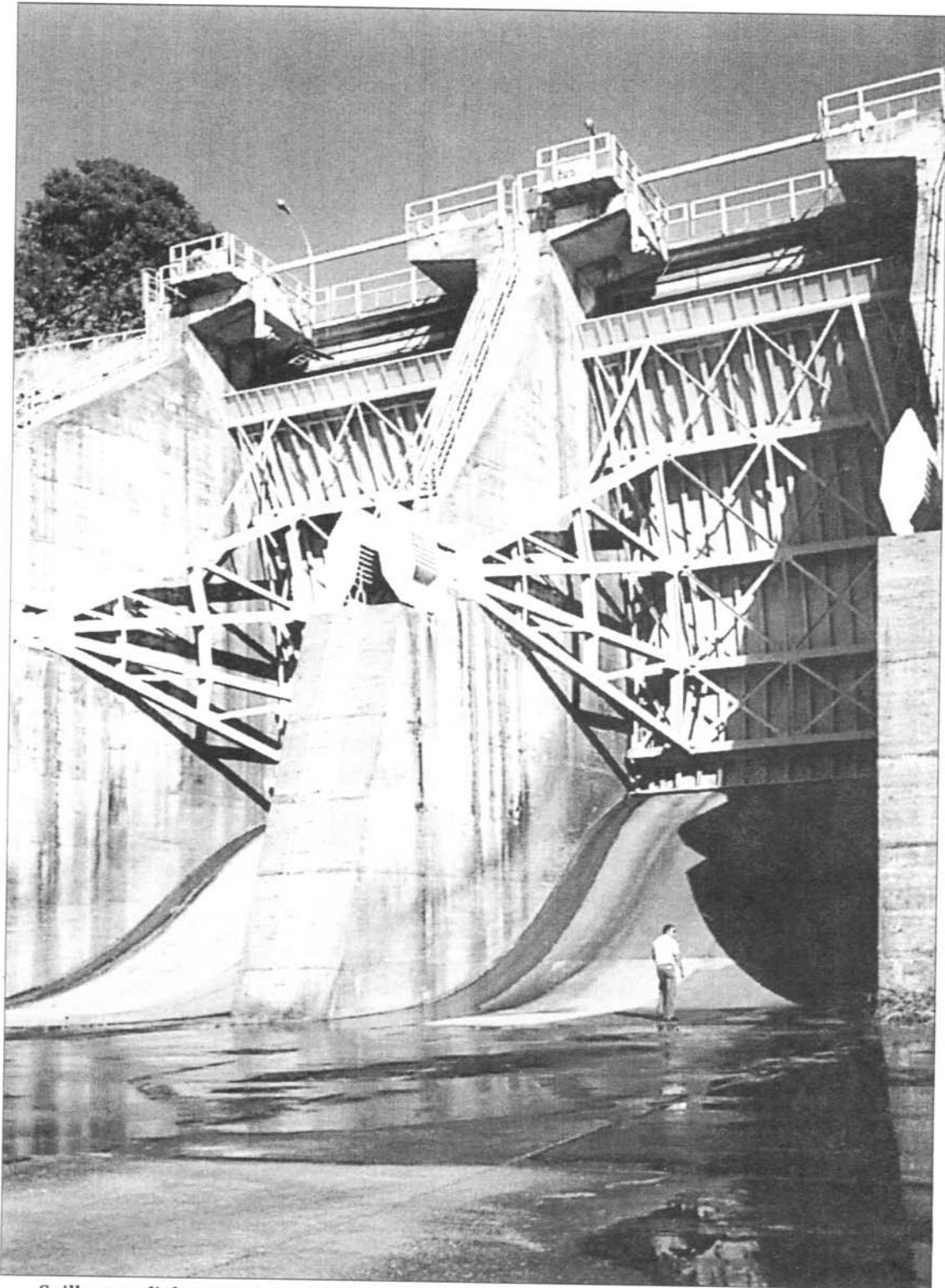
Spillway radial gates are one of the most critical appurtenances of a water resources project. Their safety and reliability are crucial. There are several factors for gate designers and project operators to consider in both operation of existing gates and design of new ones to ensure safety.
