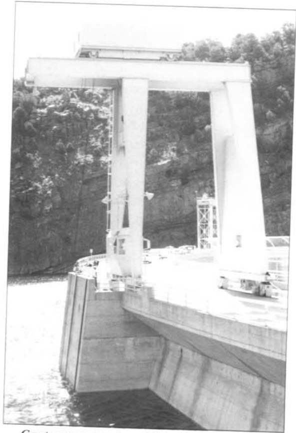
Gantry crane on top of Flaming Gorge Dam used to place the bulkhead gate in front of the opening to the damaged bypass tube.
