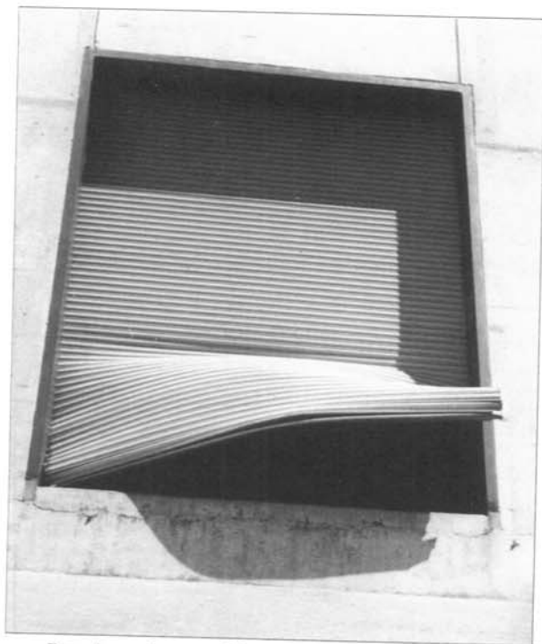
Bay door damaged by water pouring through the hole in the outlet tube.
