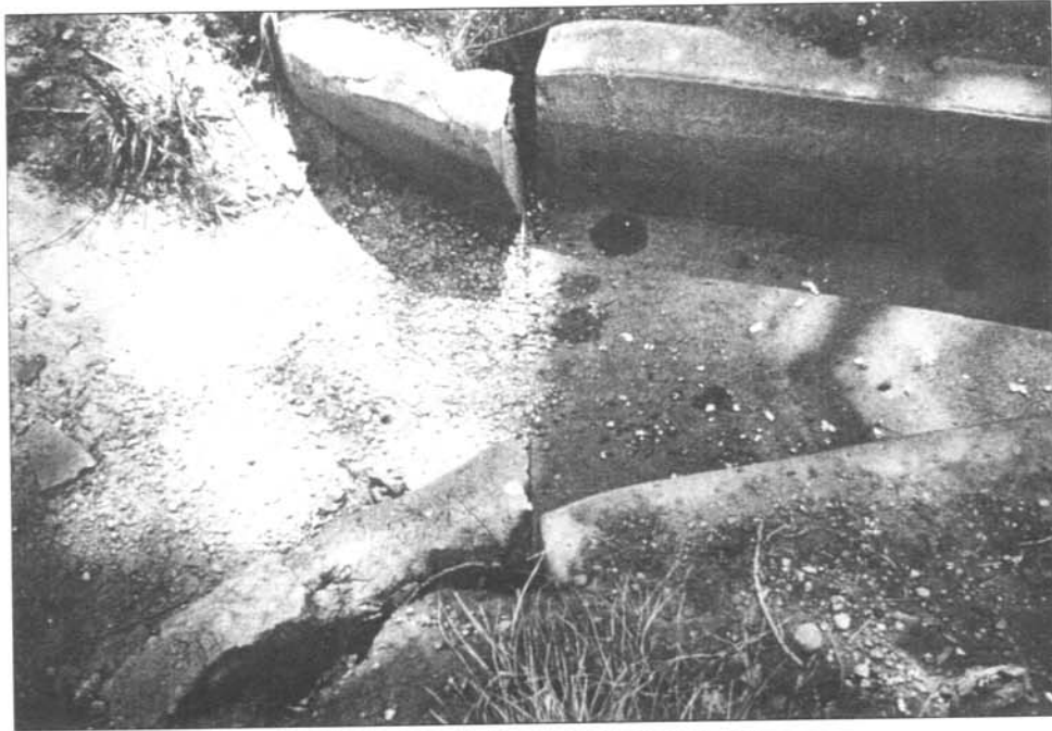
Figure 10.—Settlement at flume outlet.
