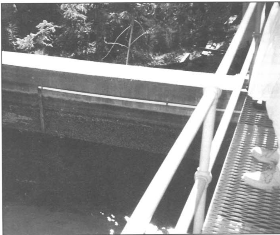
Photo 3.—Bubbler tubes attached to concrete flume.
