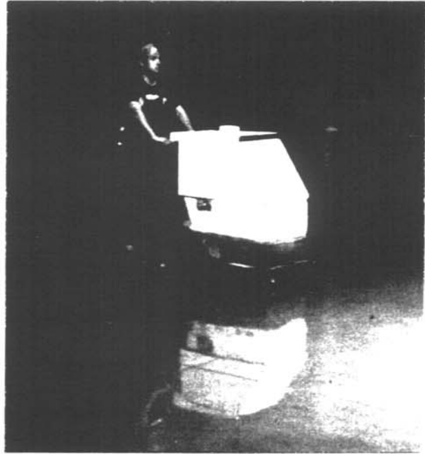
Using a buffing machine to polish a floor treated with liquid hardener results in a shiny, low-maintenance surface.
