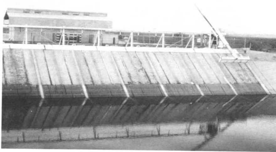
Photo 2. – When surface waters become infested with zebra mussels, the animals attach to trashracks and screens of nearby facilities. With early detection, these structures can be cleaned manually with minimum impact on operations. If mussels are allowed to build up on these structures, they impair flow; and cleaning the structures releases shells that often become a nuisance as they are carried downstream by currents.
