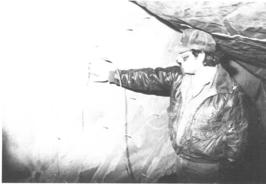
Dave Nolan of the BRID points to resin beginning to bleed from crack.
