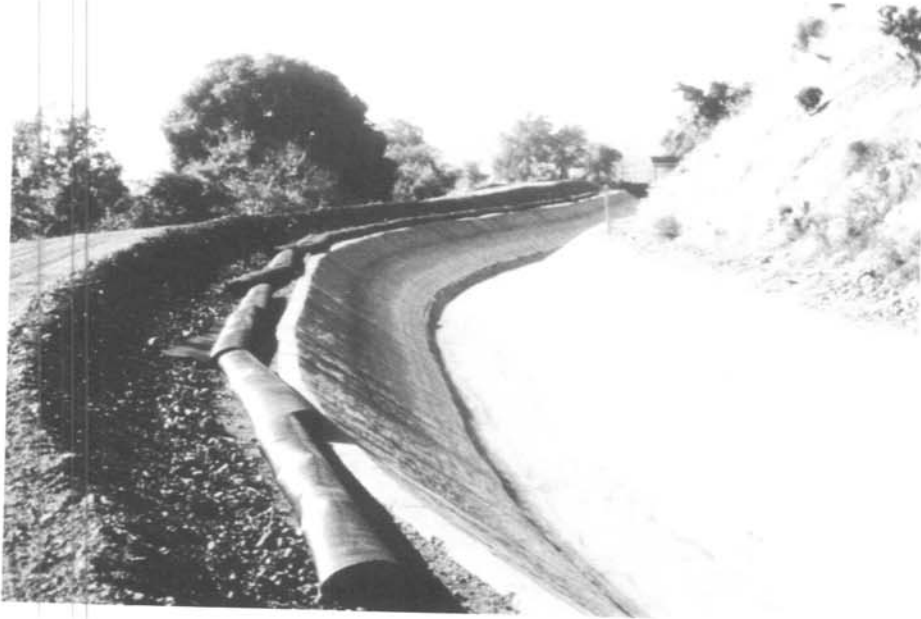
Photo 1.-Original concrete lining before repair.
