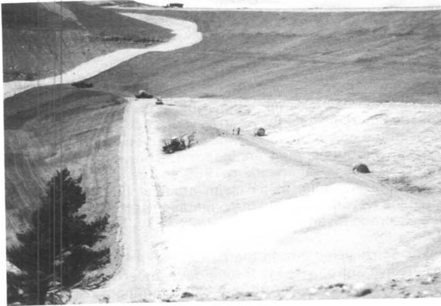
Overview of downstream slopes of Oldman River Dam. Light areas have straw spread and await crimping.
