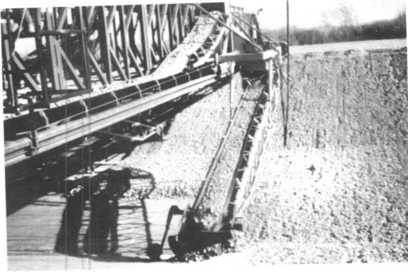
Figure 2. - Conveyor-belt system of adding protective soil cover on membrane lining. Seen following lining placement at far right of previous photograph. (Photo courtesy of Alberta Environment, Alberta, Canada.)
