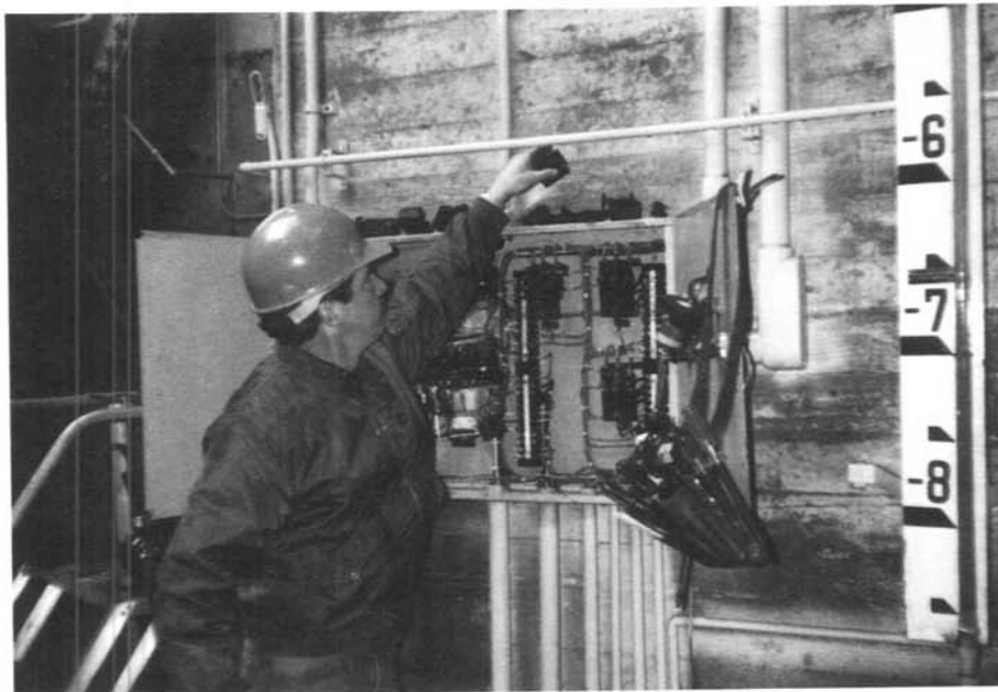
Photo 10. - Unit 4—Cleaning electrical panel that was flooded. 1/18/91
