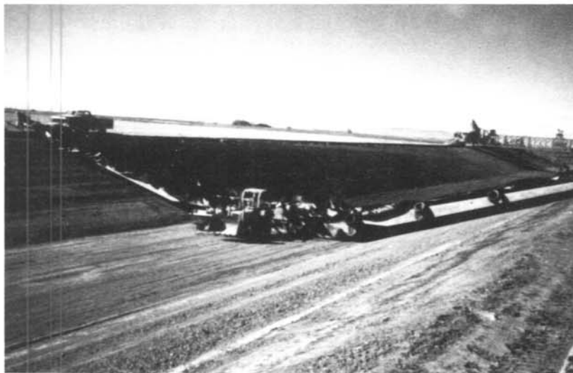
Figure 1. – The modern way of placing plastic membrane lining on equipment-trimmed soil subgrade. (Photo courtesy of Alberta Environment, Alberta, Canada.)
