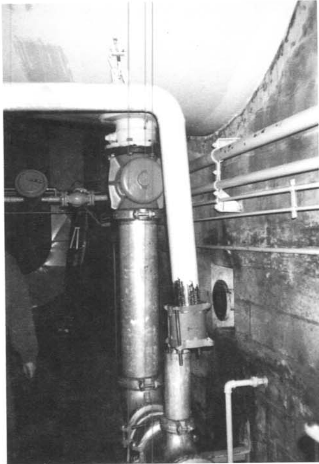
Photo 5. - Unit 6—Second sleeve coupling that separated. Note hanger at elbow does not restrain vertical movement. Vertical restraint was not needed prior to retrofitting because previous pipes had flange coupling at 10-inch pipe. 1/18/91
