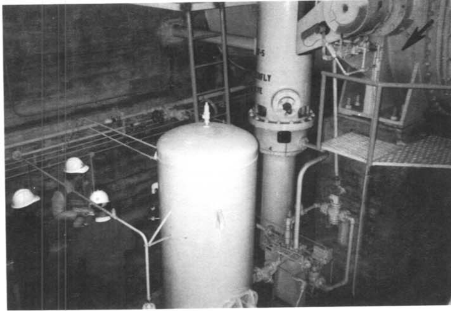
Photo 9. - Unit 5—Arrow points to oil scum line left behind as the water level receded. 1/18/91
