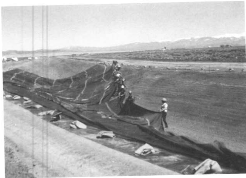
Figure 3. - An old way of spreading plastic membrane. The membrane was covered with soil by a dragline operating from the top of the bank.
