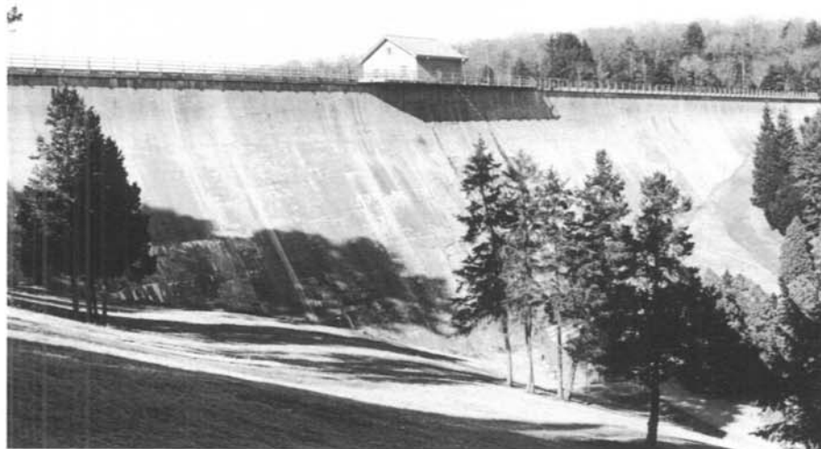
Freezing and thawing of reservoir leakage on the downstream face and ponded water on the crest of Easton Dam caused deterioration and spalling.
