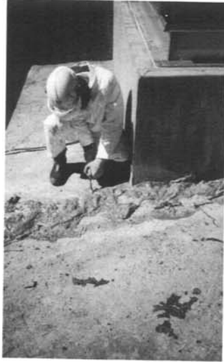
Figure 5. - Excessive resin leakage wastes material. When this happened, the contractor stopped injecting and forced resin-soaked oakum strips into the joint. This contained the foam.
