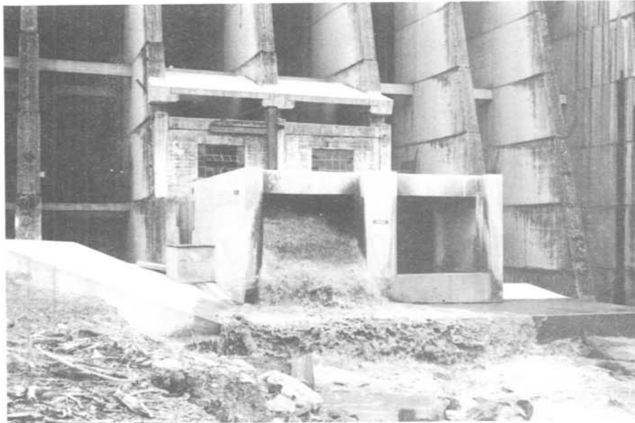
Figure 4. - Discharge from right fixed-cone valve flowing from the energy dissipation chamber. Photo by Bill Bouley. 10/26/89.
