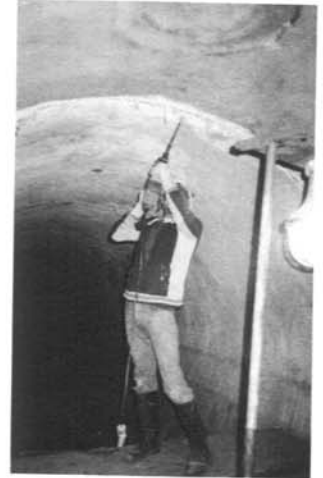
Figure 6. - Workers also drilled and injected resin into holes inside the water tunnel. Resin injected from the outside of the tunnel portal extrudes from the joint.
