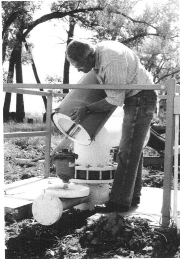
Technologist, Paul Ewashen, demonstrates how easily an insulated canister can be removed for valve inspection.
