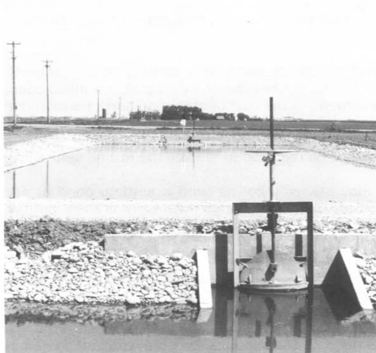
The settling pond constructed in 1989 on the SMRID's Coaldale Lateral is lined and gravel armored.
