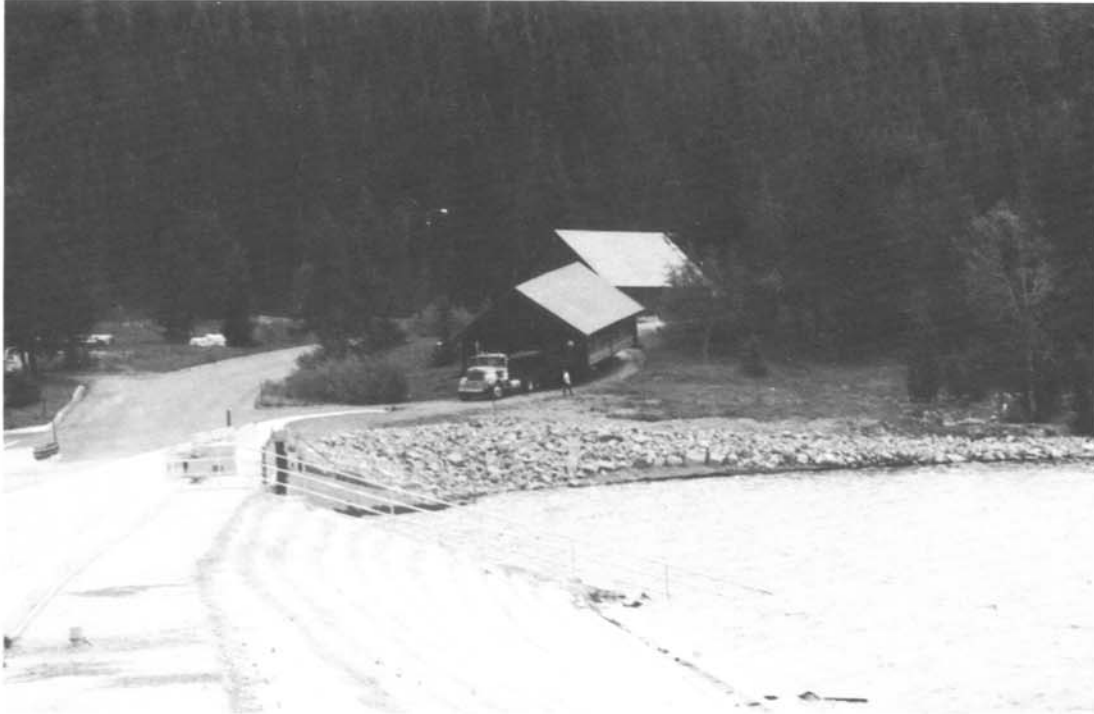
Photo 5. - View of warehouse building being moved from the old Reclamation maintenance area. This area will be turned into a parking lot, and the building will store boats at Colter Bay. — Bureau of Reclamation photo by S. Bareis. 6/26/89
