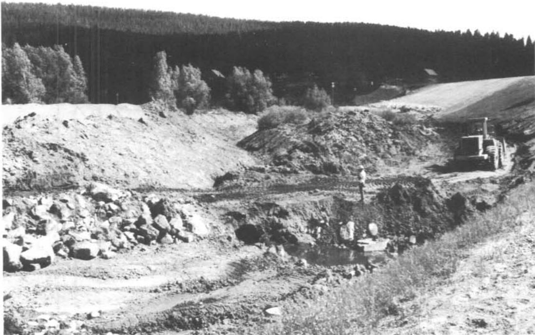
Photo 4. - The photo shows subcontractor constructing a new drainage ditch and rebuilding the embankment of the Teton Park Road to a 2.5:1 slope. Stockpiled fill material is at left, new ditch and temporary CMP at center, and alignment of old ditch (beneath loader) is at right. — Bureau of Reclamation photo by S. Bareis. 6/29/89
