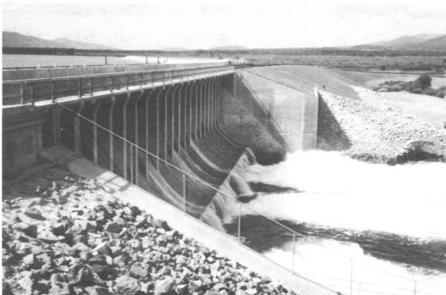
Photo 6. - Jackson Lake Dam discharging about 1,610 ft 3 /s through the outlet works. — Bureau of Reclamation photo by Bill Bouley. 7/27/89
