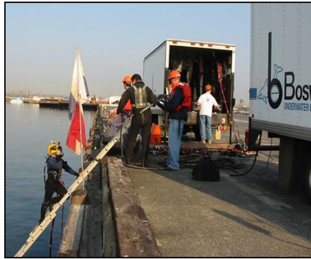
Based on OSHA and Coast Guard guidelines, an underwater inspection carried out in a confined space environment would warrant a dive team comprised of six persons.
