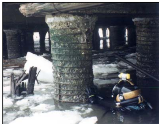
Inspection divers must be sufficiently trained and experienced to perform meaningful inspections in harsh environments.
