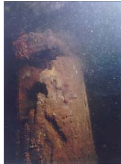
Timber pile exhibiting severe section loss caused by Limnoria attack.
