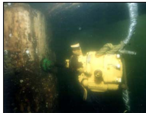
A Level III inspection effort on a timber substructure will often include destructive core sampling of piles to evaluate the extent of marine borer infestation.
