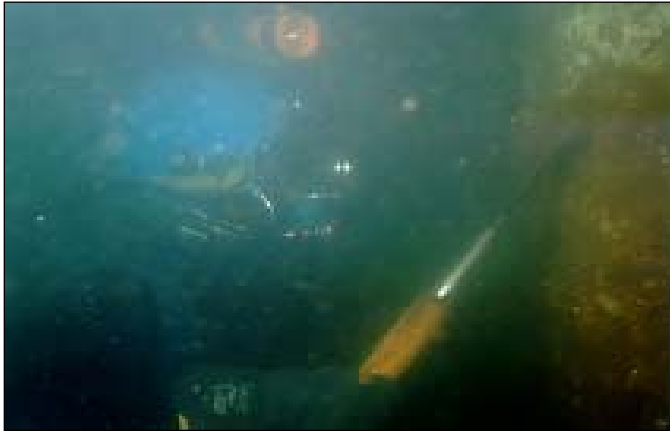
A Level II inspection effort requires partial cleaning of marine growth or other fouling encrustations from portions of the substructure to reveal hidden deterioration. Here, a diver used a hand scraper to remove barnacles from a timber pile prior to measuring its circumference.
