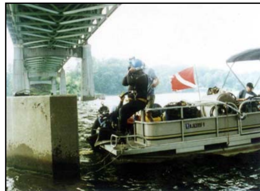
Frequent diver changeovers are important when adverse conditions exist to avoid burnout and to ensure the quality of the inspection.
